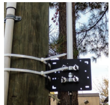
Telephone Pole Mounted Mast Antenna with GB06
