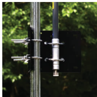
Pole Mounted Mast Antenna with GB06
